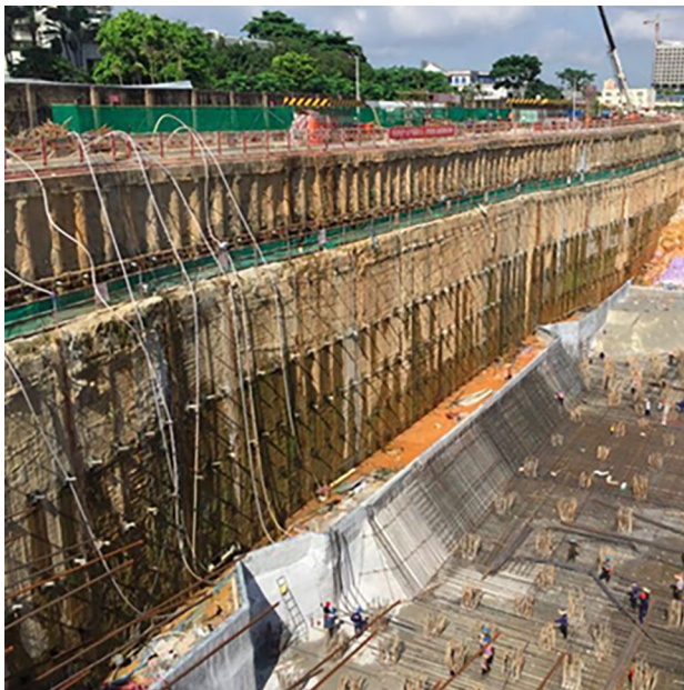
Figure 4. Construction photo of the composite retaining and protection structure at the south side of the excavations
